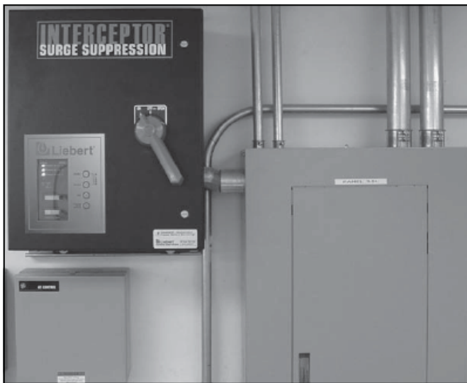
Main or Secondary Electrical Panel Example TVSS Install
